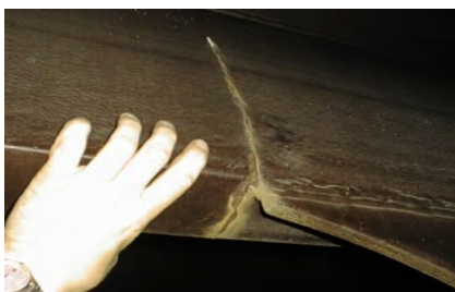
Crack in stiffener
